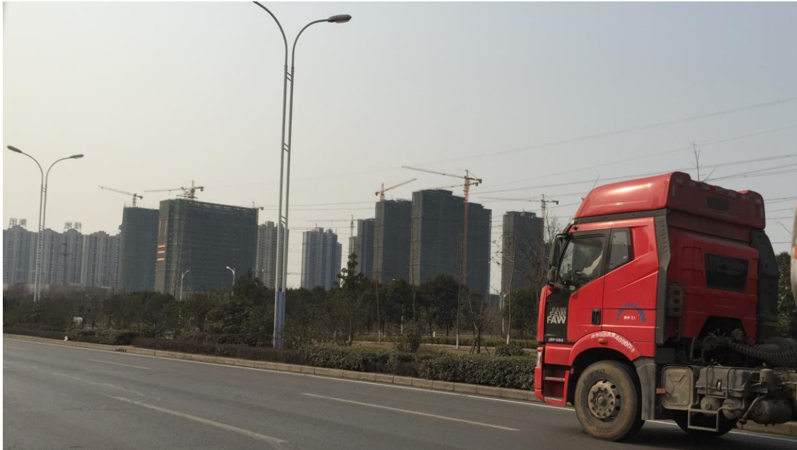
Multiple high rise apartment tower blocks & shopping malls under construction in Xiangyang City, Hubei Province, China
